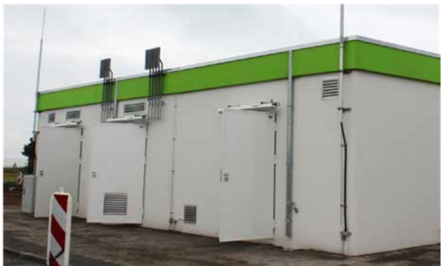
Abb. 7: Wall and pipe mounting: Internally routed isCon ® arrester in air-termination rod in biogas plant
